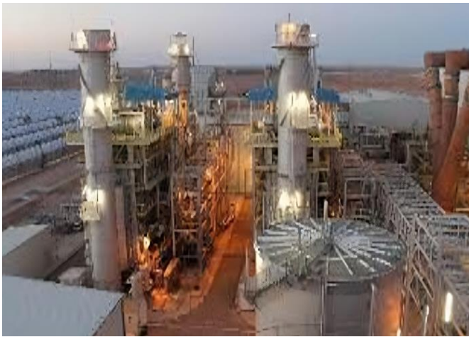
Figure 1. Solar power plant 1 in Laghouat, Algeria (ABENGOA, 2023)
